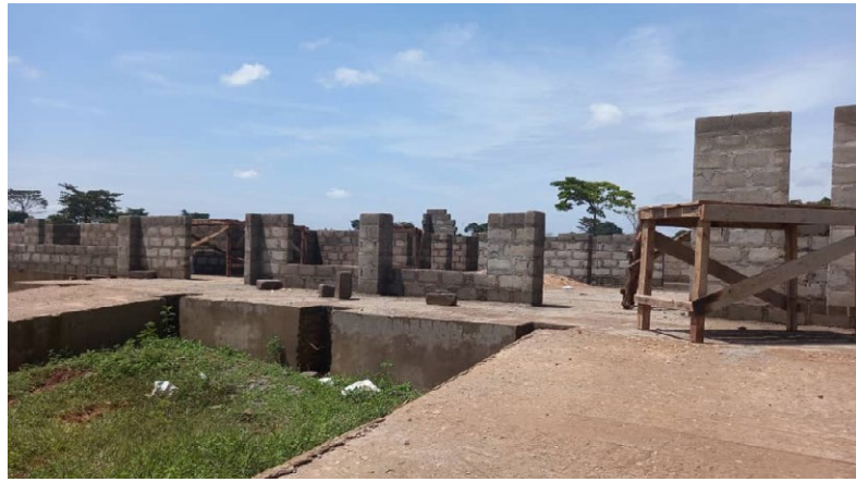
The Rotary Club of Muyenga Tankhill is constructing Tankhill Health Centre IV in Gwembuzi Village, Luuka District, Eastern Uganda, as part of their commitment to supporting underprivileged communities by addressing their most pressing needs.
