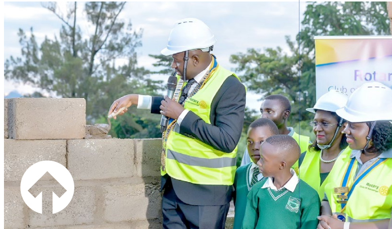
RC Kansanga constructed a classroom to manage congestion and provide a more conducive learning environment in the lower section of Kansanga Primary School.
